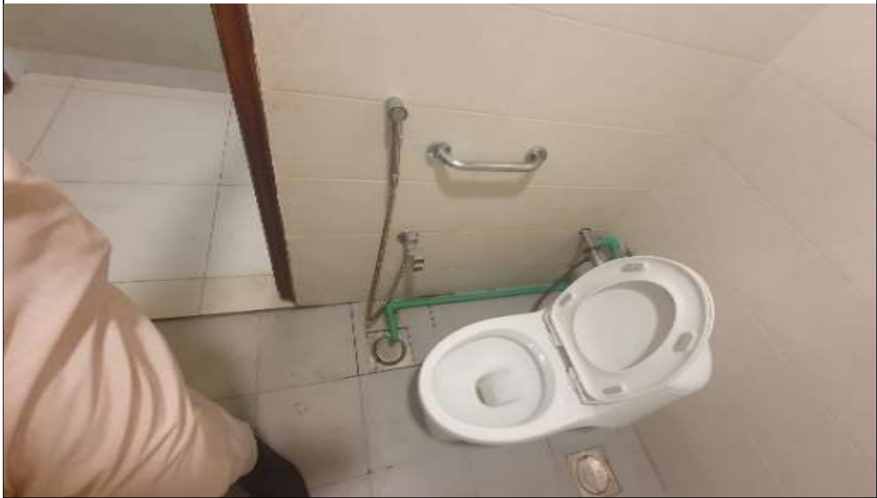
3. Toilet Seats for Disabled Persons
